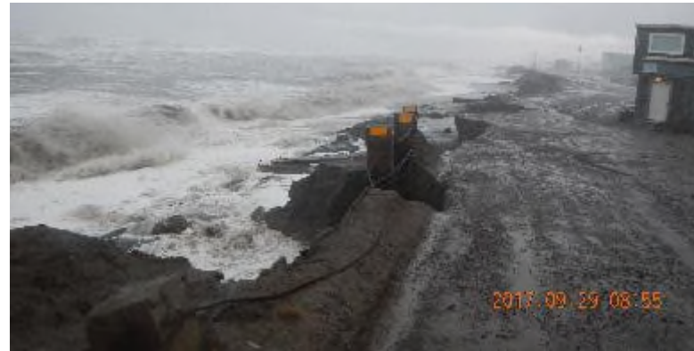
Erosion along a road during a storm
